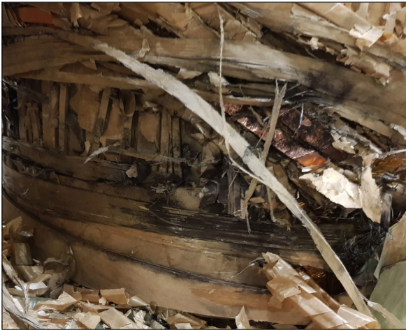
Figure 8: Phase C regulating winding as found during visual inspection
